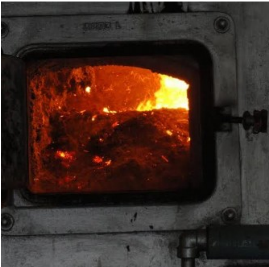
A biomass boiler. Image: FDC Enterprises
